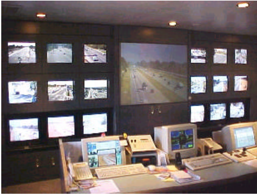
Figure 2: ACHD Traffic Management Center
