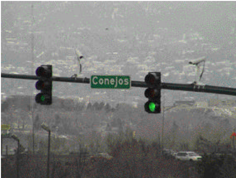
Camera on mast arm.
